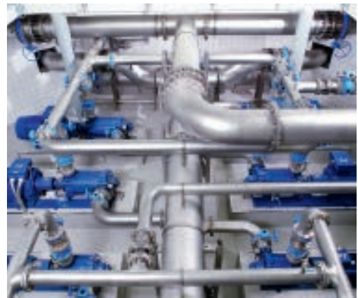
Distributed pumping stations are networked to each other and data is thus exchanged via easyNet.
